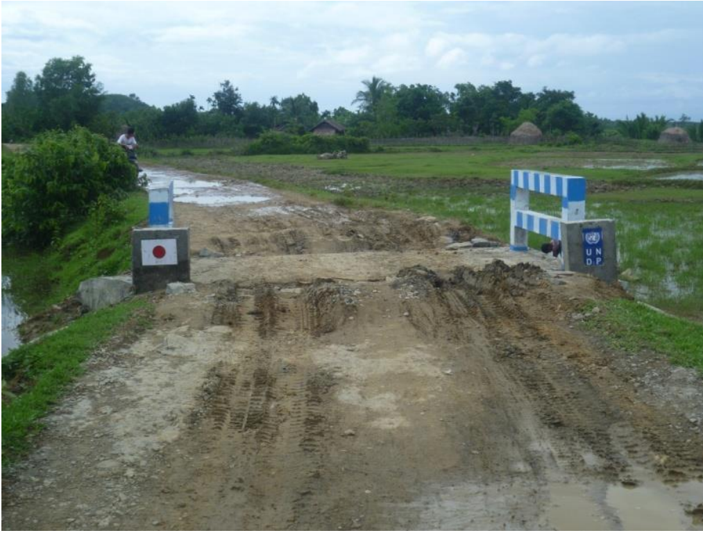
Bridge and Road Construction in Cheik Taung Village of Minbya Township (Rakhine State)
